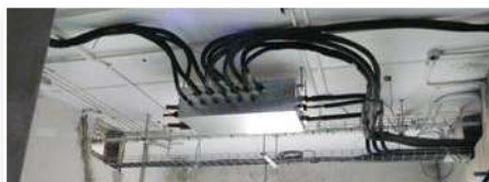
MCU boxes involved in heat recovery
